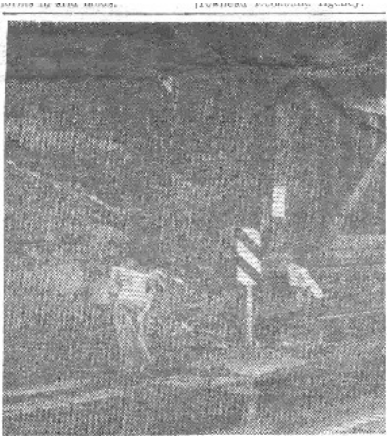
ALMOST FORGOTTEN was the damage done by the rain during the storm, as workmen from the Minnesota Highway Department repair a washout at the bridge north of Virginia on Highway 169. (MDN Photo)
